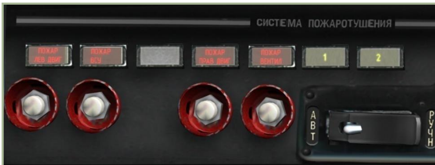
10-19: Fire extinguishing system control panel
